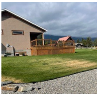
An otherwise reasonably well mitigated property, the weak points are the grass within 1.5m of the home, especially where it meets the highly flammable wood lattice and the wood deck. Embers may also accumulate in the window well, or on the deck itself.
