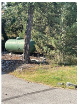
High density, high flammability vegetation in close proximity to propane tank. Vegetation should be removed.
